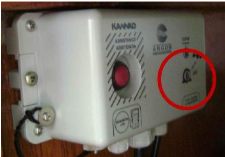
Figure 84: Argos junction Box switched off
