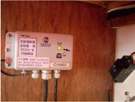
Figure 66: Argos junction Box with on/off switch
