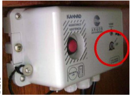
Figure 67: Argos junction Box switched off
