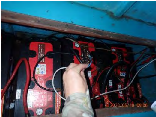
[Fig 40] BlueTraker VMS ConBox 2018 LCD cut off from electrical power.
