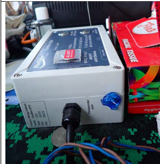
[Fig.9] VMS not functional
