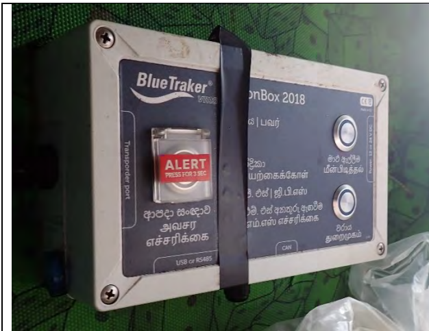
[Fig.7] VMS not functional
