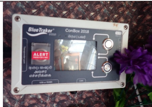
[Fig.28] VMS not working (vessel's batteries or alternator issue reported by captain).
