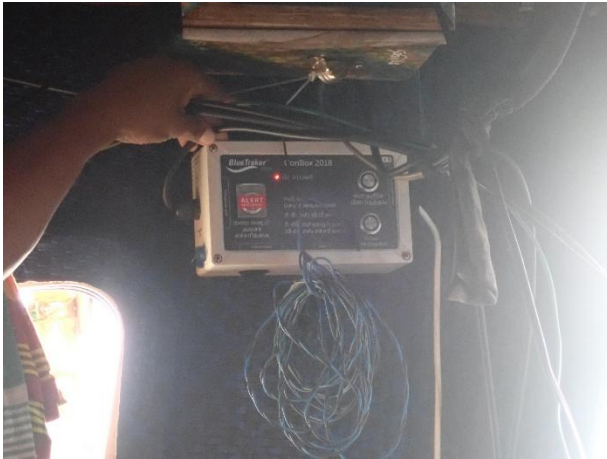
[Fig. 30] VMS BlueTraker ConBox 2018, not operational. Red light blinking, connection between the transponder and ConBox not established.
